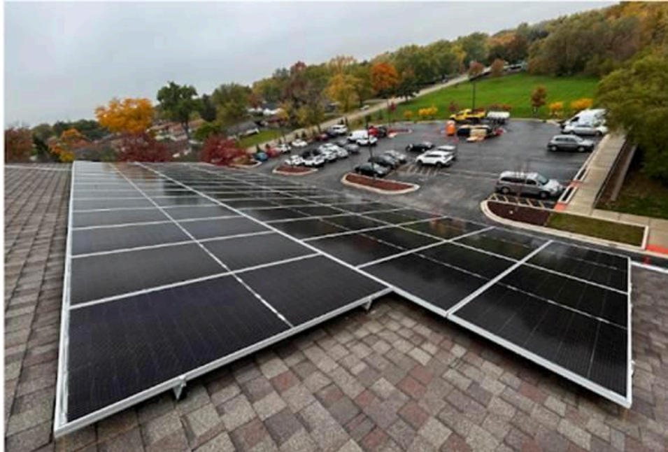
Figure 5: Schaumburg Township solar array
