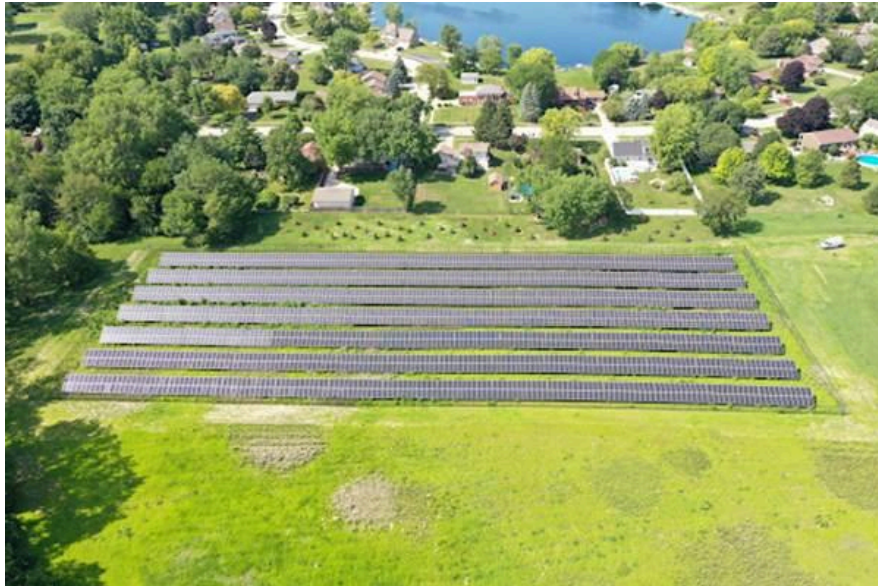
Figure 2: Village of Minooka WWTP ground-mount array.
