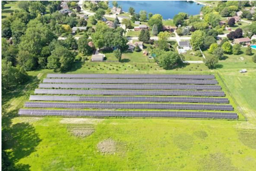
Figure 2: Village of Minooka WWTP ground-mount array.
