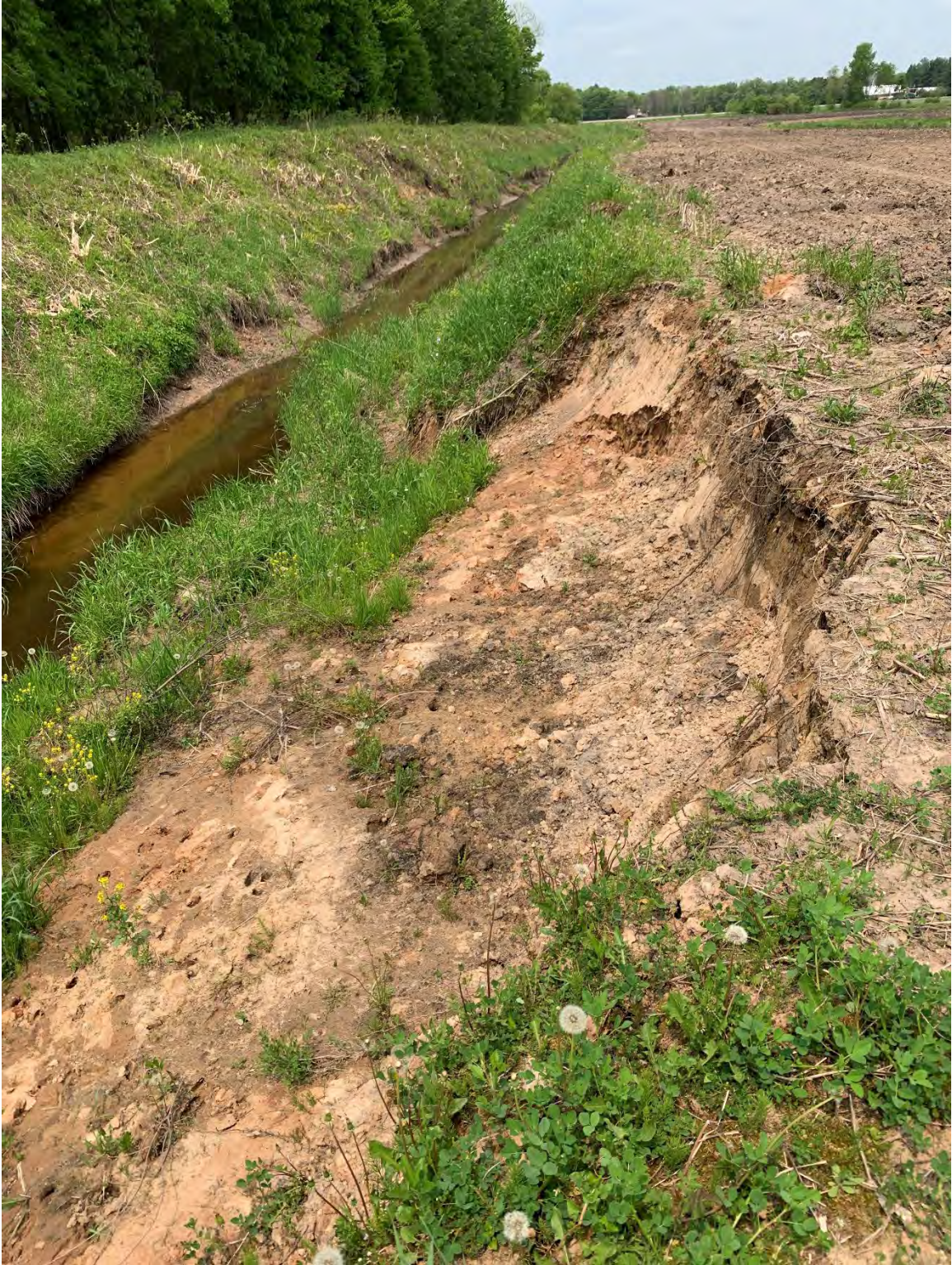
Schrock bank failure, view looking north
