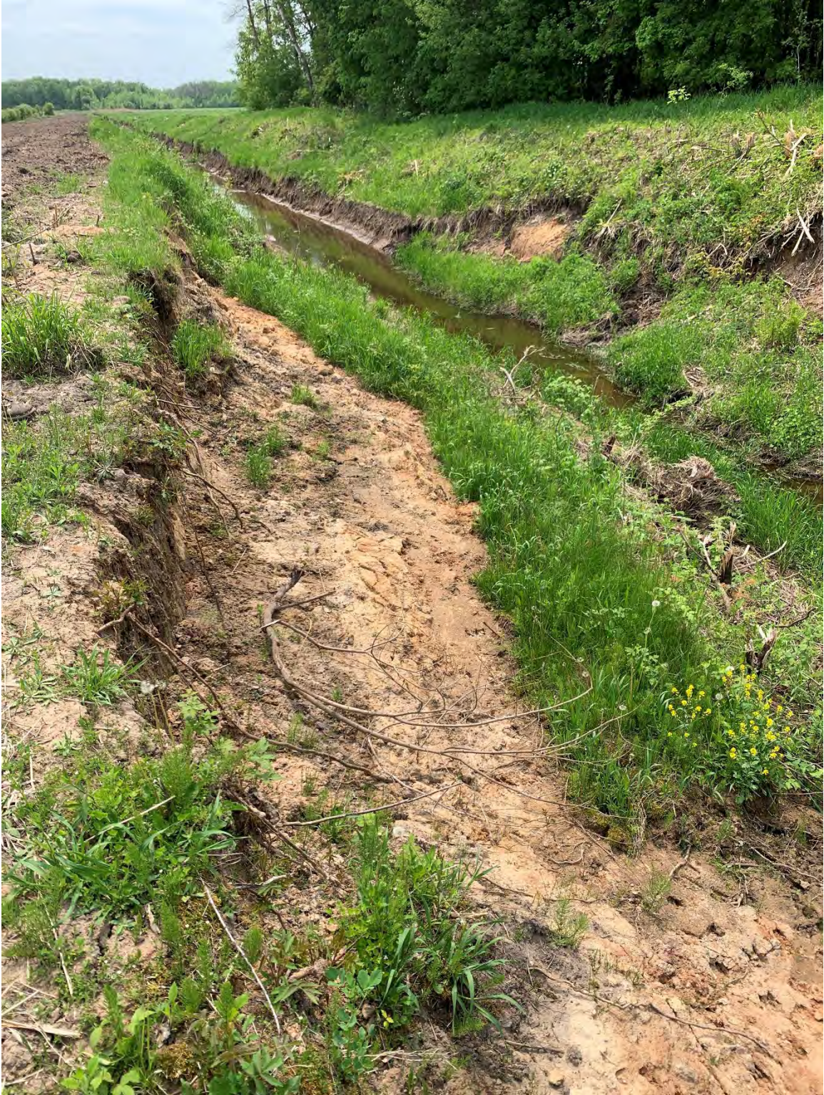
Schrock bank failure, view looking south
