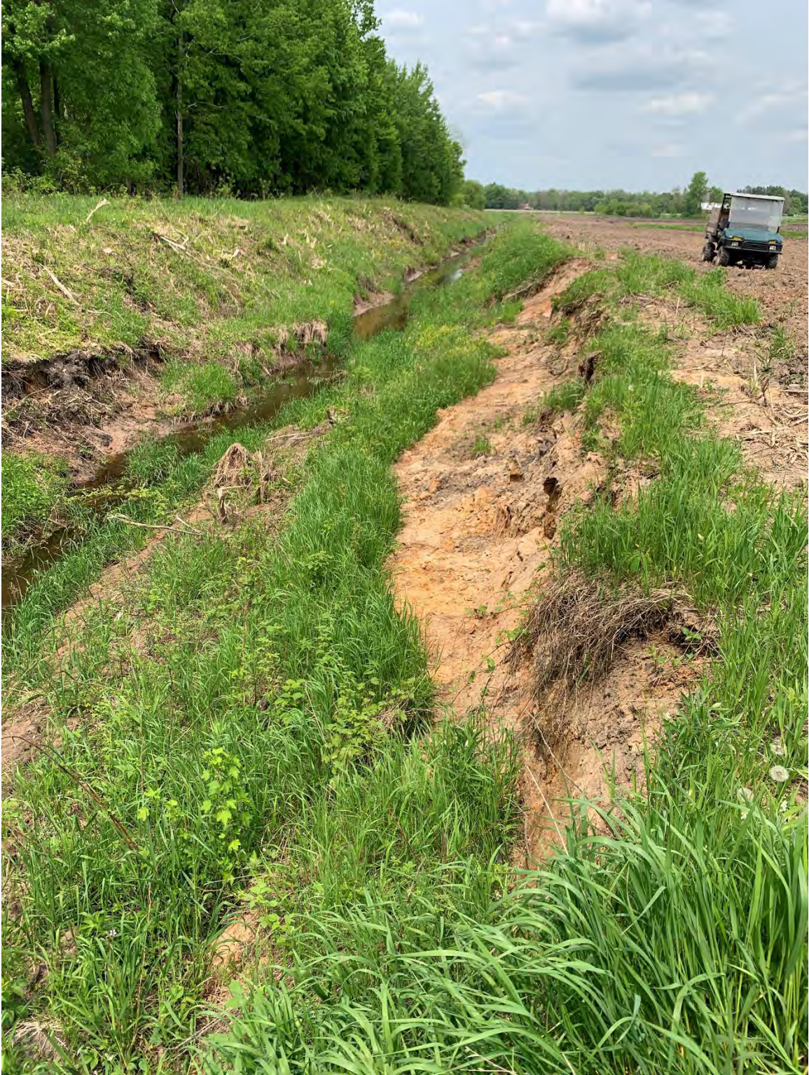
Schrock bank failure, view looking north
