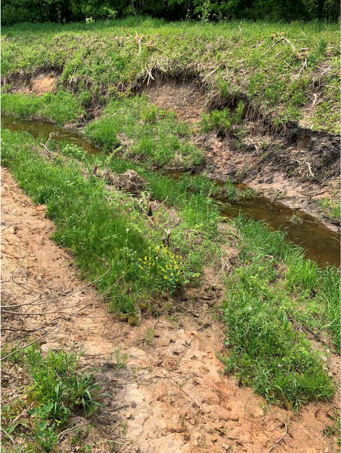
Schrock bank failure, filling in channel
